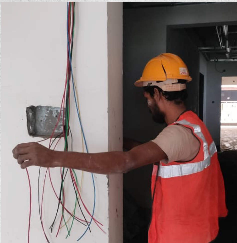
Wiring and installations of switch boards.
