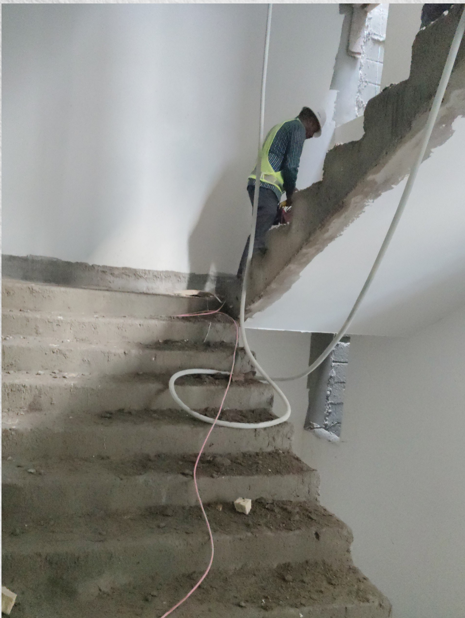
Staircase steps are chipped and cleaning works in Progress.
