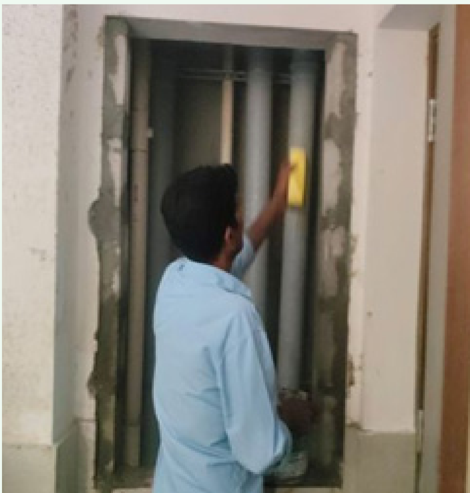
Plumbing soft pin plastering works and UPVC window bottom plastering works are currently in progress in the Flat No. 1 series.
