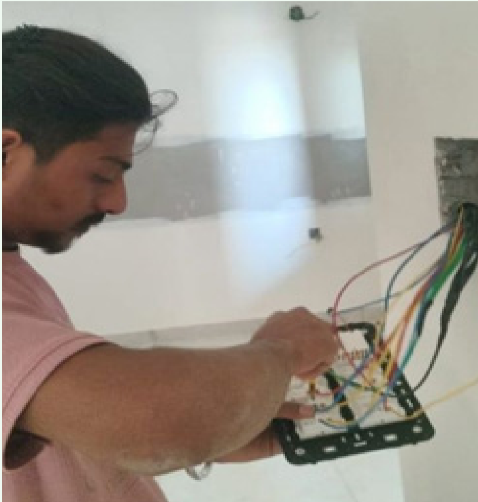
Electrical switchboard connection works are currently in progress across the flats in Tower 4.
