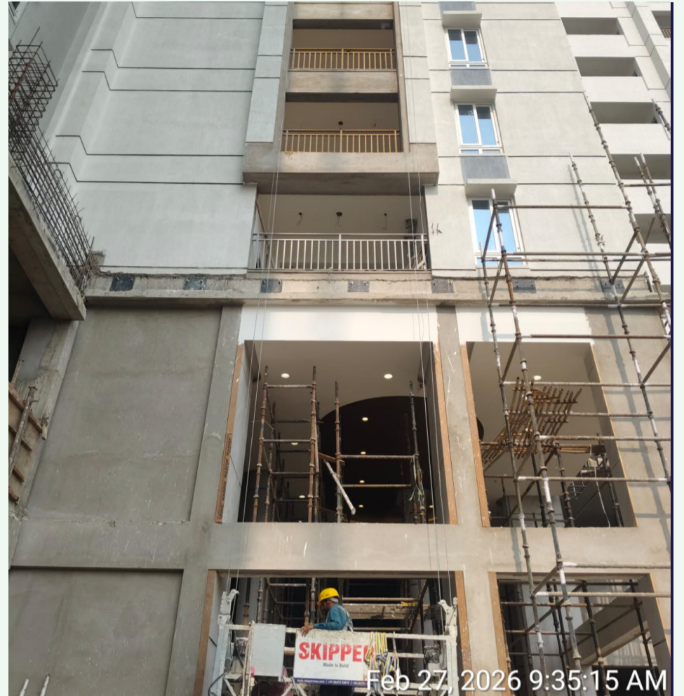
Bottom plastering works beneath the granite at east-facing living room balcony of a flat - In Tower 4 are underway.
