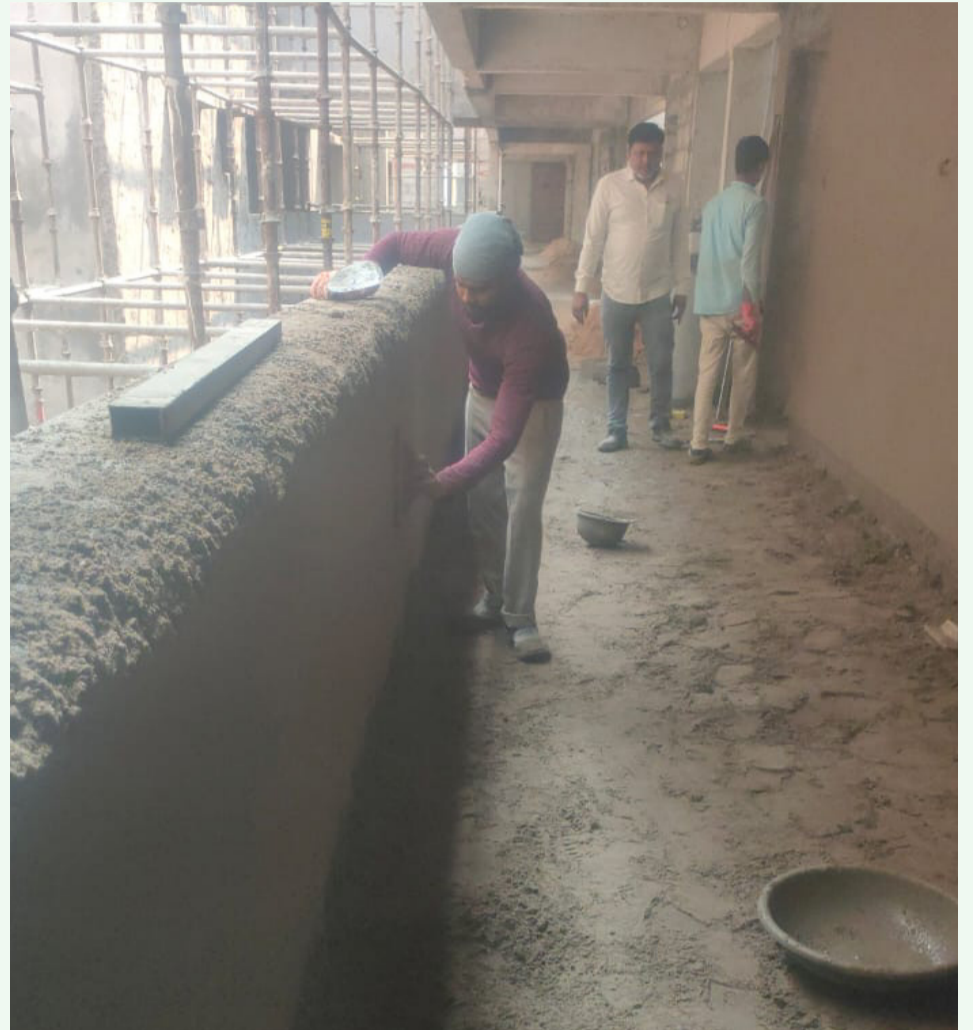
Plastering works in the 11th floor corridor area are presently in progress.
