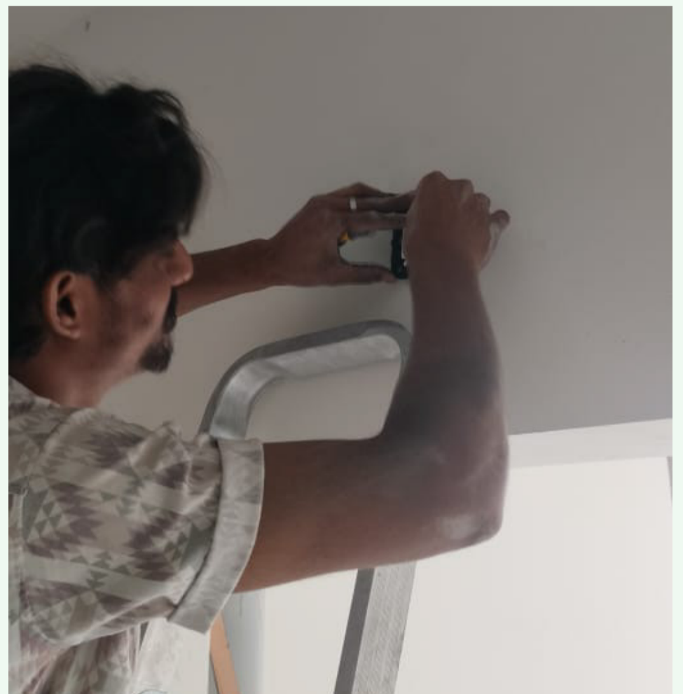
Installation of Switch Boards in the flat no .1 series is in progress.
