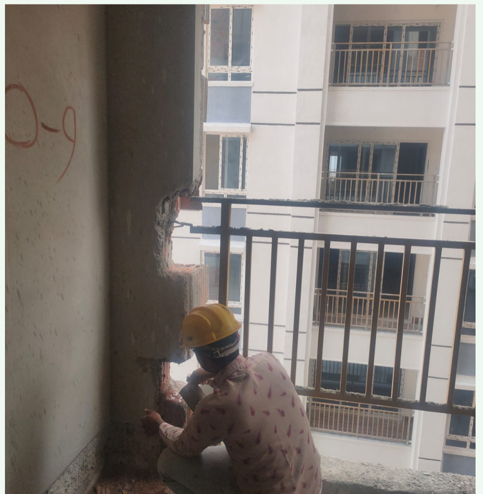
Railing protection and packing activities are in progress in Flat No.1 series.
