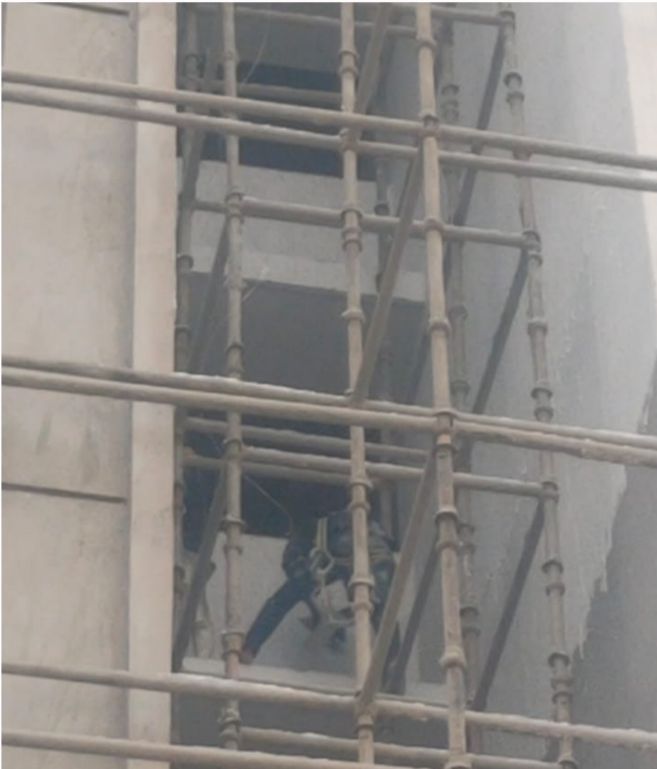
Texture application for the OTS on the north side, covering the 11th and 12th series, is currently in progress.
