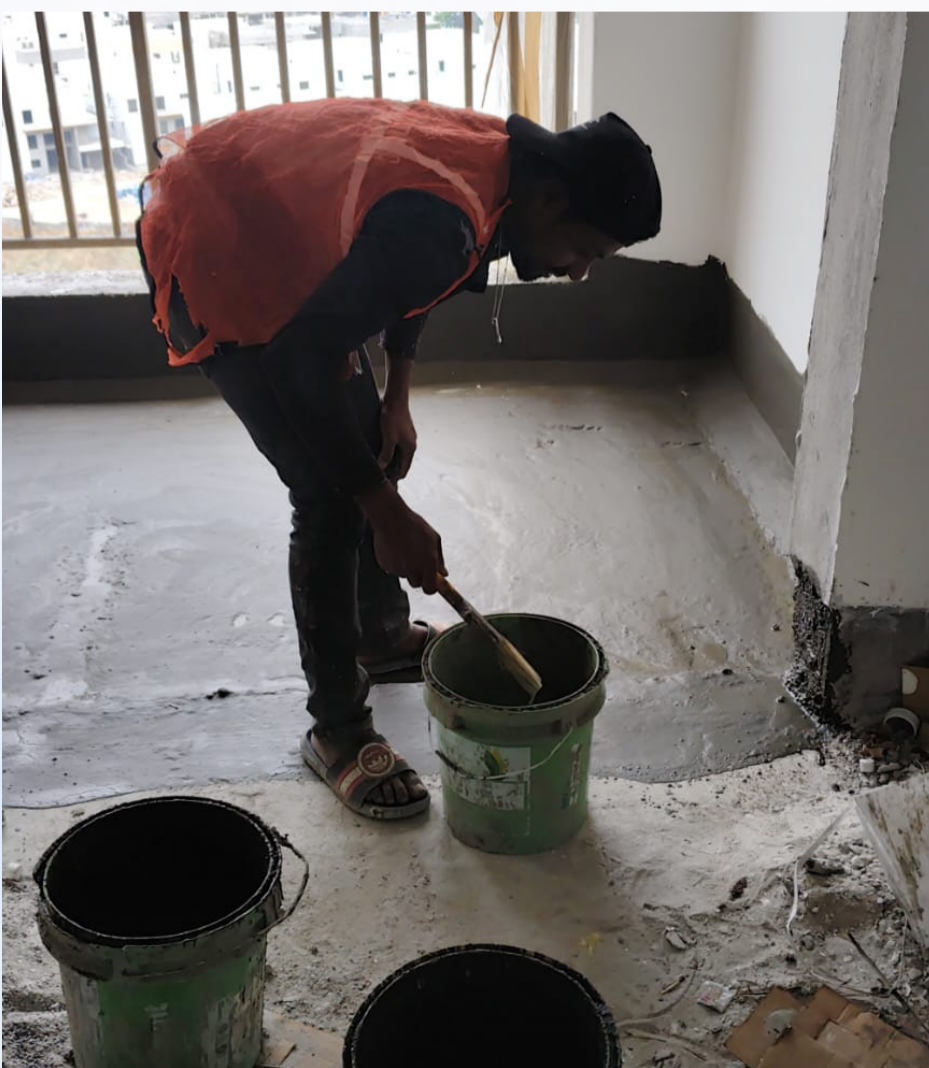
Application of two coats of CP in the 9th floor sit-out area is currently in progress.
