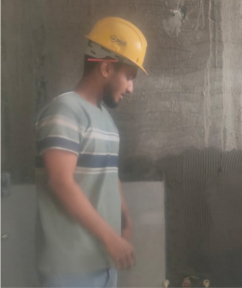
Cladding tile fixing work in the master bedroom toilet of the 8 Series is currently in progress.
