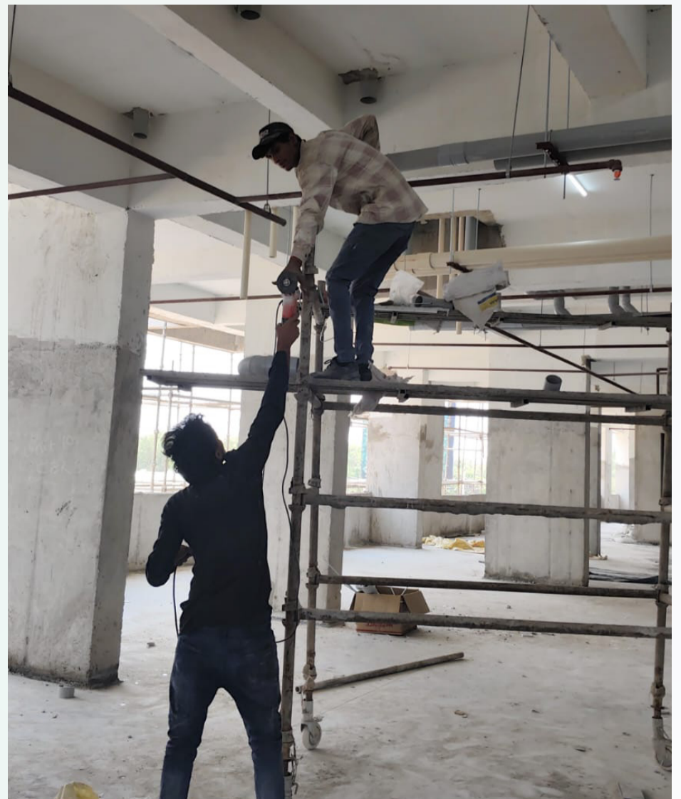
PVC main waste line work at P-2 level is currently in progress.
