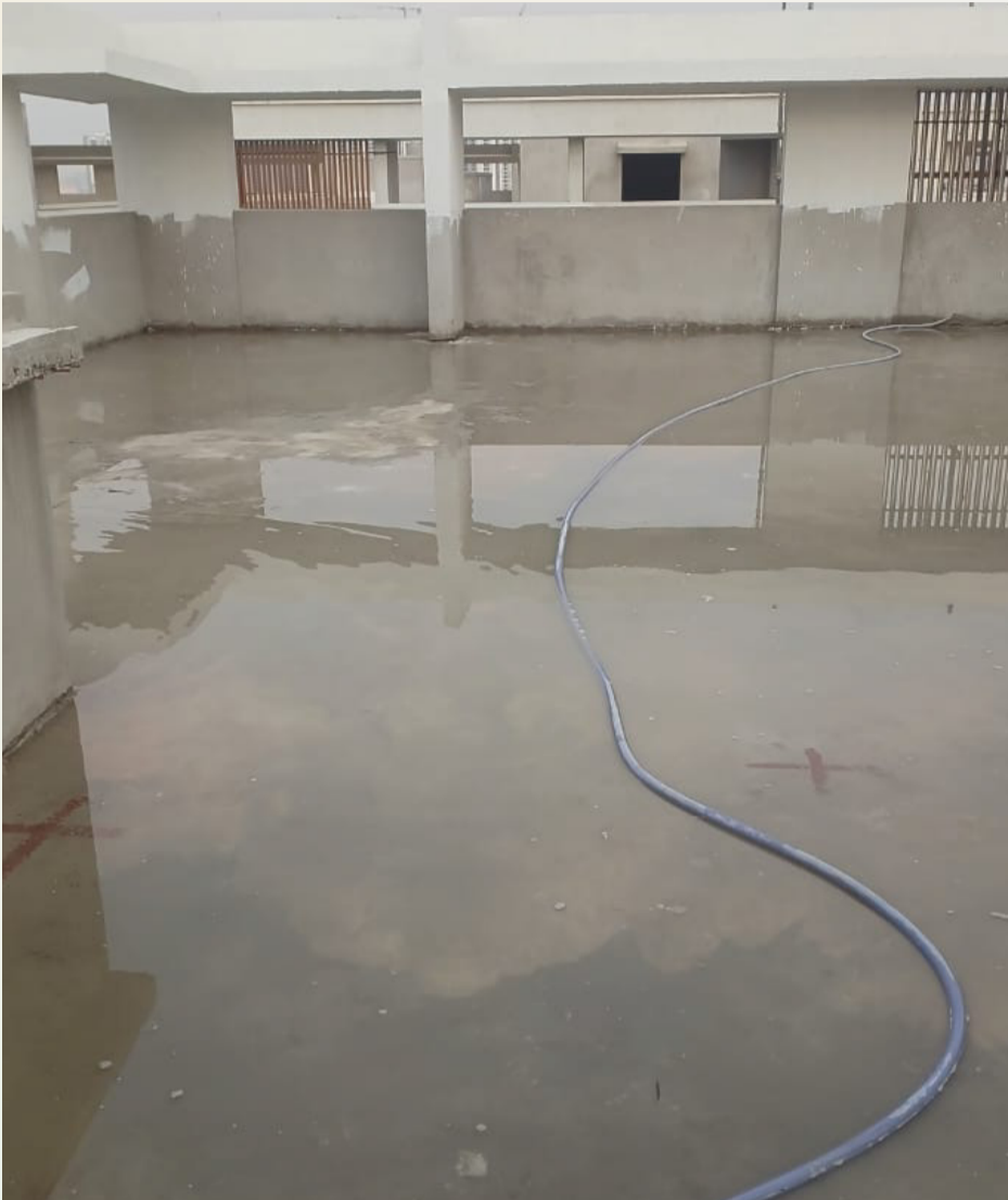
Series No. 2, Terrace Area: Water Pond testing in progress for Flat 1202 handover
