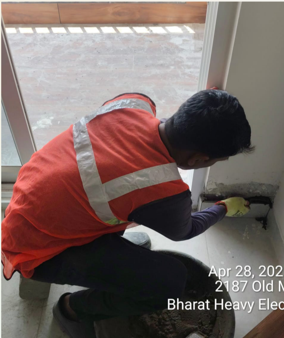
12th Floor Flats: Door frame side skirting top plastering work in progress,
