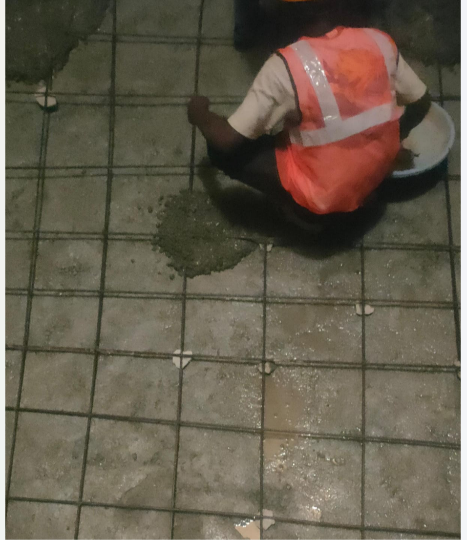
RCC laying work for the service lift pit is currently in progress.
