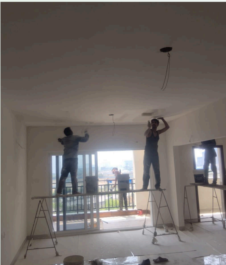
Second coat painting for rooms and MS railing works are in progress ahead of customer handover.
