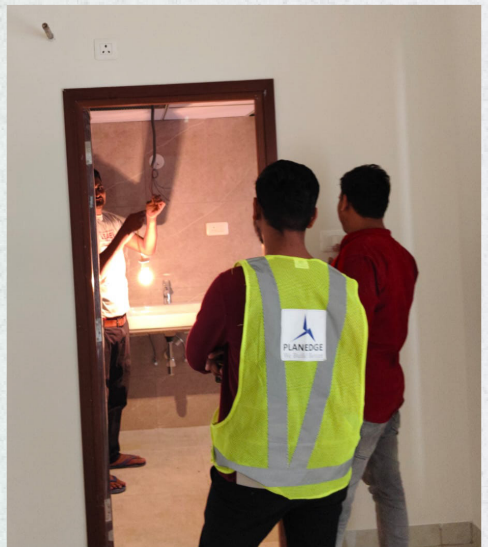
Third-party MEP snagging inspection is in progress.
